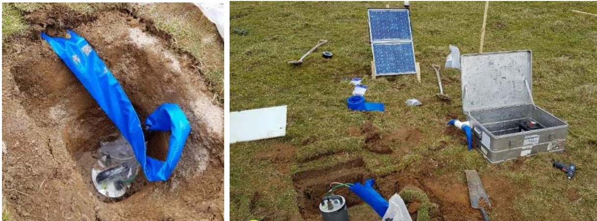
Figure 2: Left: Typical 6TD installation at the HHLO site. Right: Wider station setup showing solar panels and customised storage box for housing battery, data disk and cable connection box.
