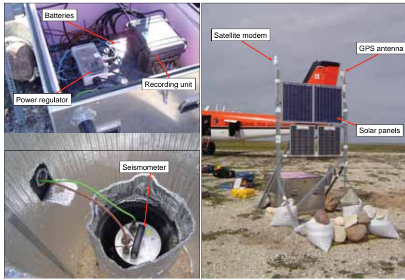
Figure 2: HuBLE-UK remote station construction. 20-40W solar panels on a steel frame re-charge 3x100Ah batteries that power the seismometer and recording equipment. The GPS antenna provides continuous accurate timing information for our data. We communicate with the stations remotely via the satellite modems that are scheduled to operate twice weekly. After Bastow et al. (2011a).
